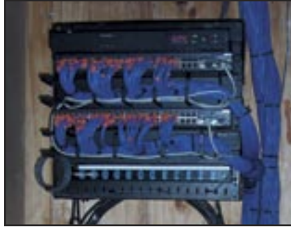
Figure 1. Simple, straightforward MDU building demark. The bandwidth comes in on fiber.
